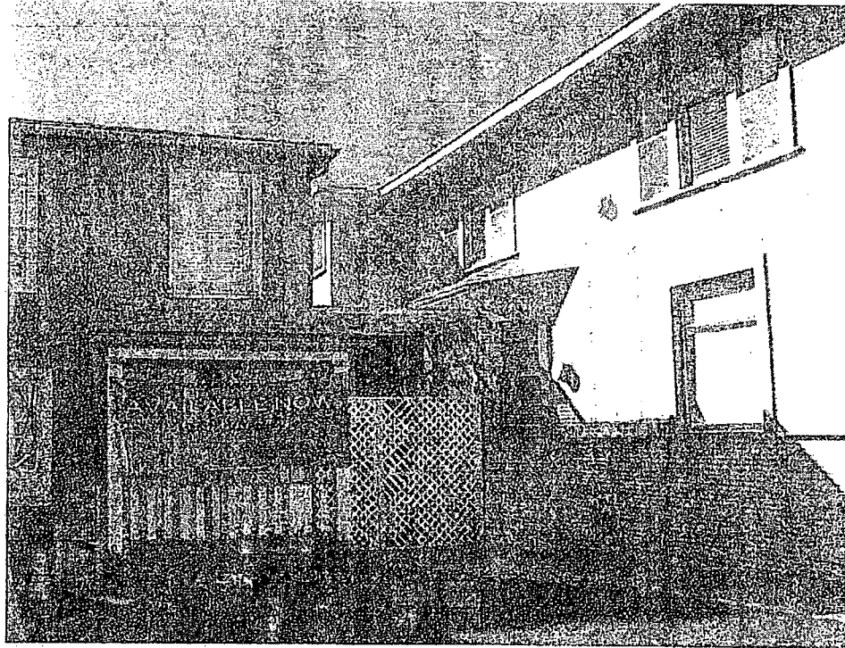
View of the south façade of 3616-3618 4th Avenue. The two-story addition is behind the lattice fence.
