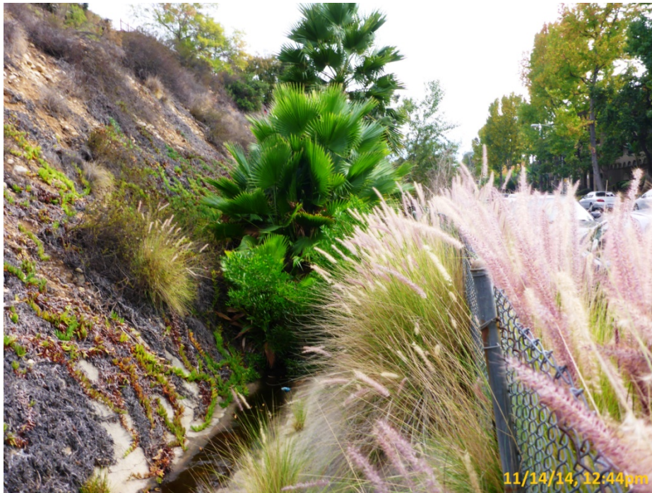
Photo 9: Reservoir Drive Channel Emergency Pre-Maintenance 11/14/14
