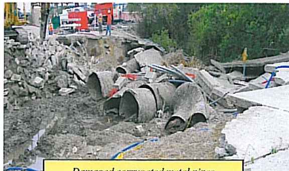
Damaged corrugated metal pipes
